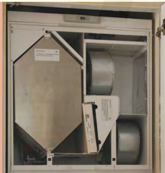
Ventilation unit with heat recovery
