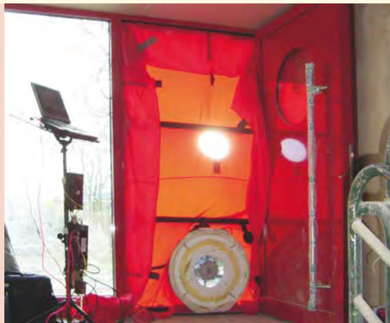
Fan for pressure test
